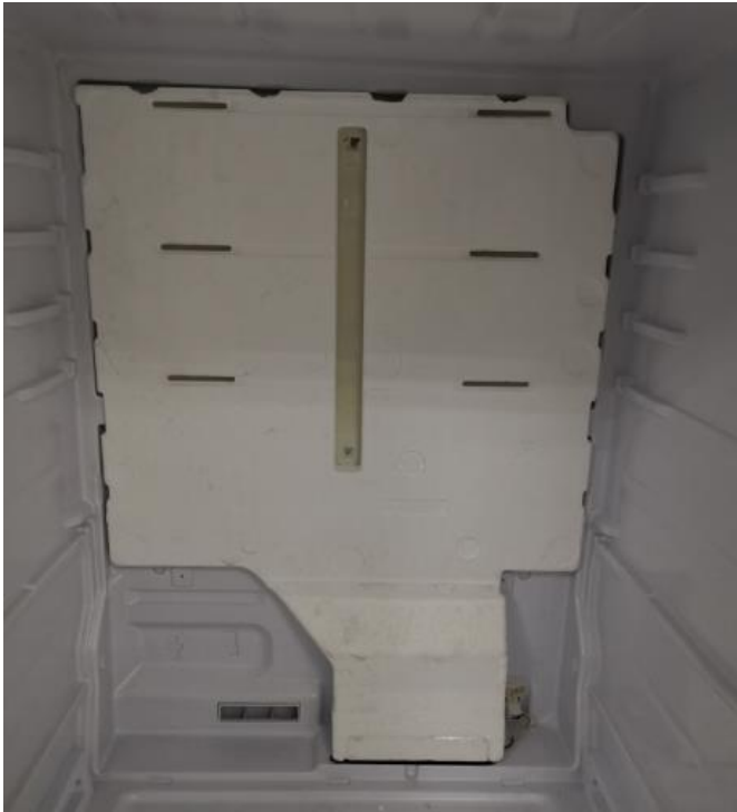
Refrigeration room air duct
