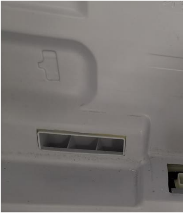
Refrigeration room back to the air vent
