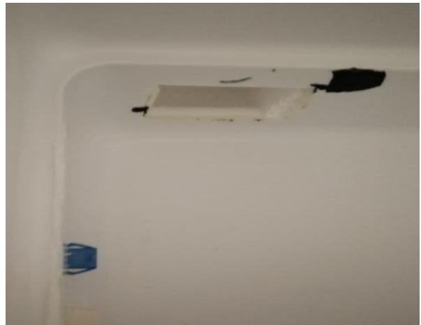
Freezer → air supply outlet of fridge
