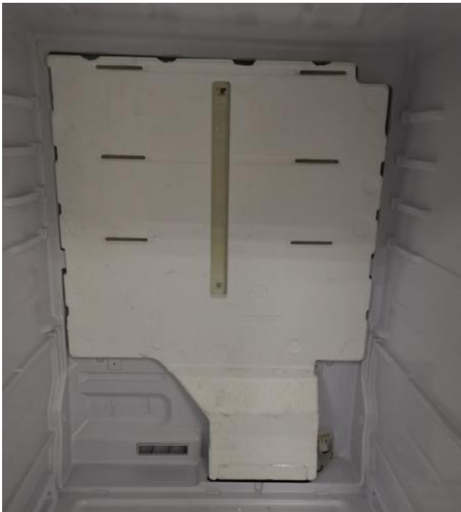
Refrigeration room air duct
